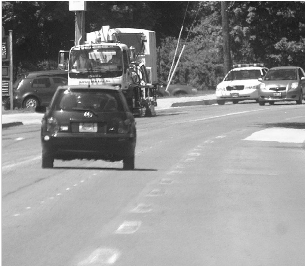
The R.I. Department of Transportation was busy last week preparing a section of Bristol Ferry Road in Portsmouth for a lane reduction.
