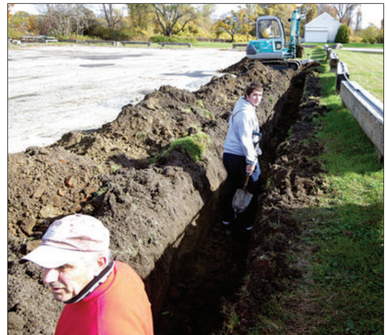
Volunteers have been making improvements to the Legion Way ice rink for years. This work, digging a trench to install wiring for new lights, was conducted in 2010.
