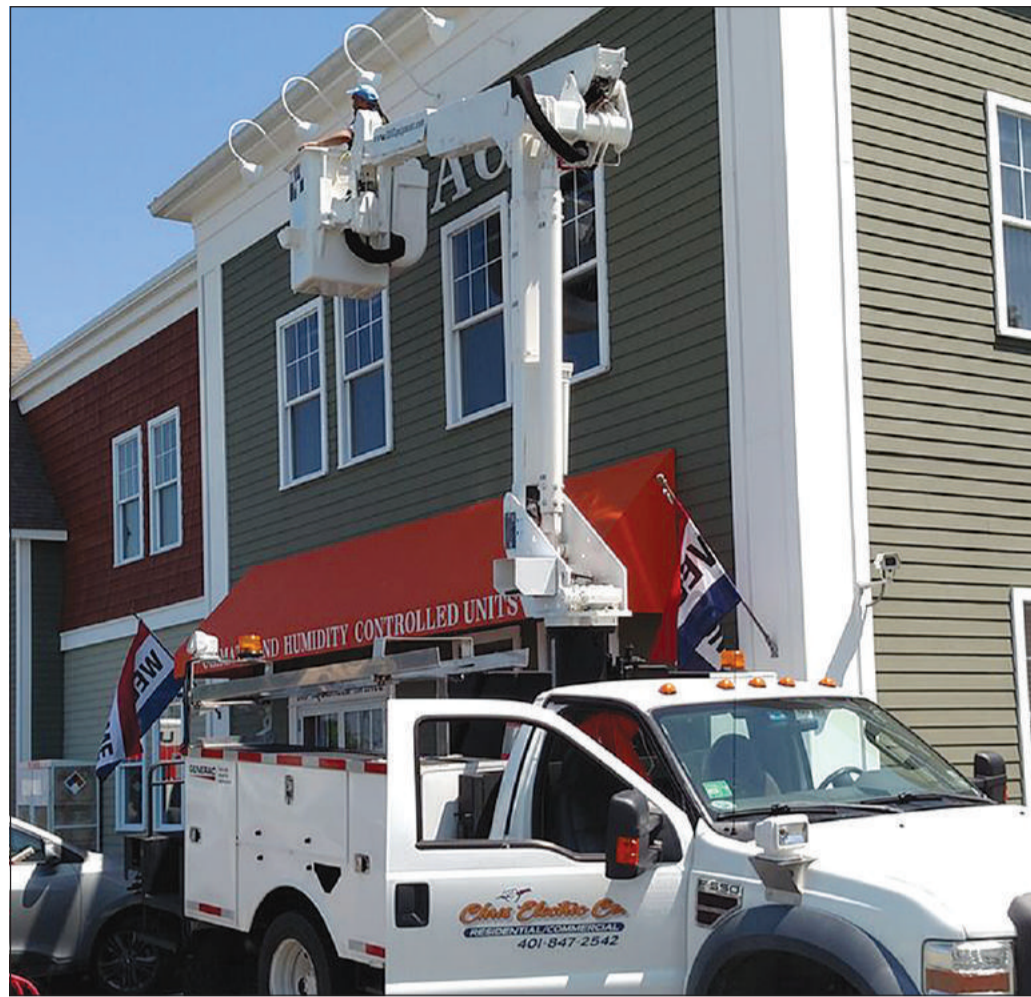
The Chris Electric crew can handle any job, from smart-home wiring to installation of generators, from home renovations to commercial upgrades.
