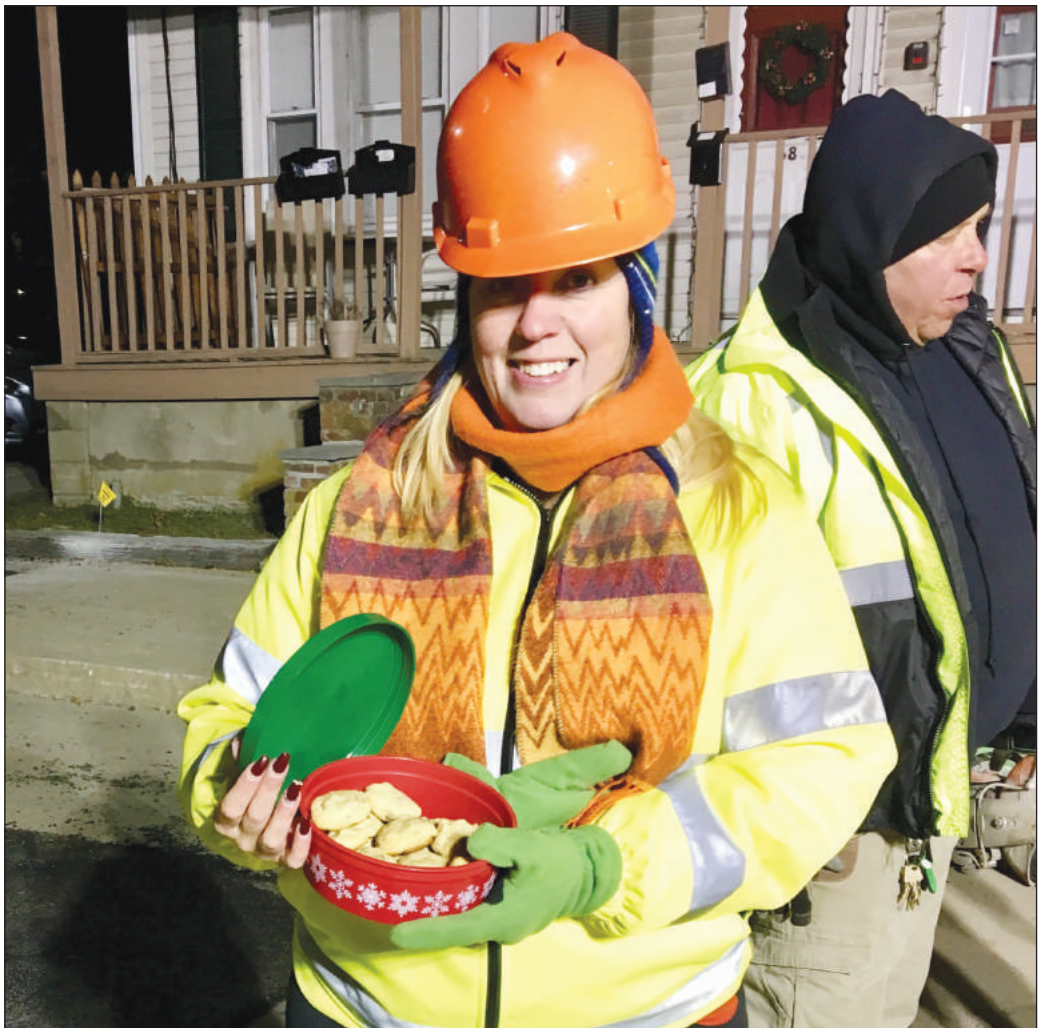
ABOVE: Workers on the site of an emergency repair on Wood Street last Friday evening. LEFT: Warren Town Manager Kate Michaud and the crew shared a bash of fresh-made chocolate chip cookies, brought out fresh from the oven by neighbors.
