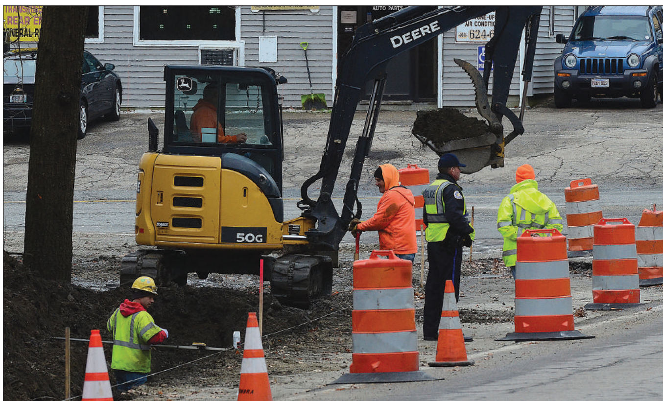
Crews prepare the intersection of Bulgarmarsh and Fish roads for the new light.
