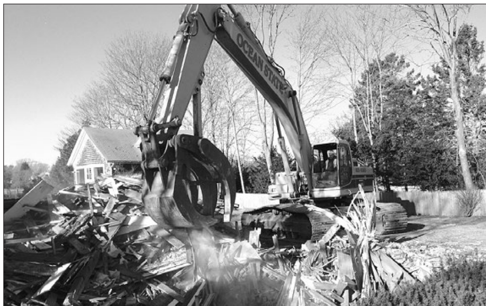
On Thursday morning, Dec. 12, all that remained of the James Bowen House was a pile of rubble.
