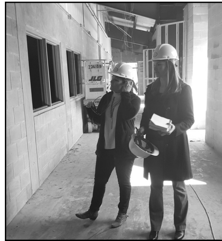
McLaughlin and Ellis survey a hall under construction at Discovery Oaks Elementary.
