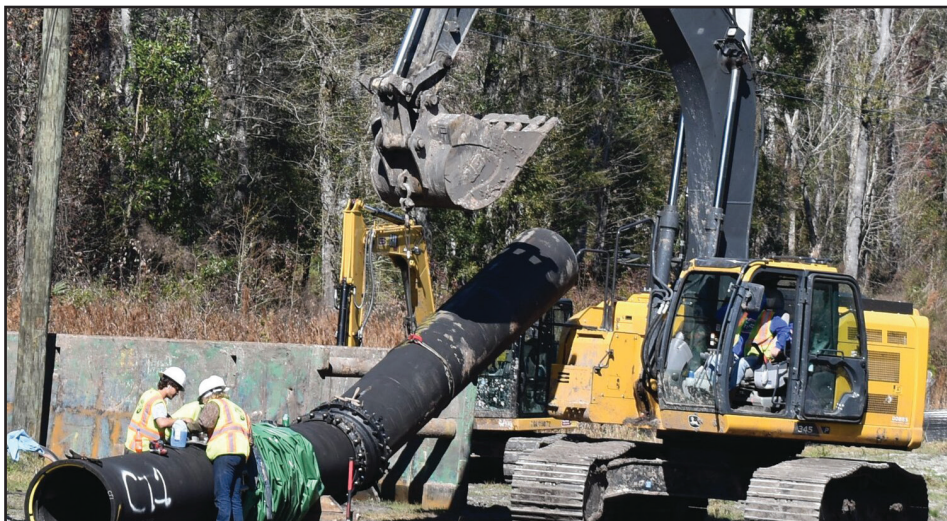
Construction crews have stayed on schedule building a pump station and drain field at South Fork of Black Creek in Green Cove Springs and installing 17 miles of pipes that will siphon as much as 10 million gallons, which would replenish lakes Brooklyn and Geneva in Keystone Heights.
