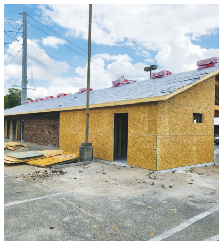
The remodeling of the Pizza Hut in Starke continues. Gary Park hopes to soon have his former employees working at a new G's Slow Smoked BBQ.
