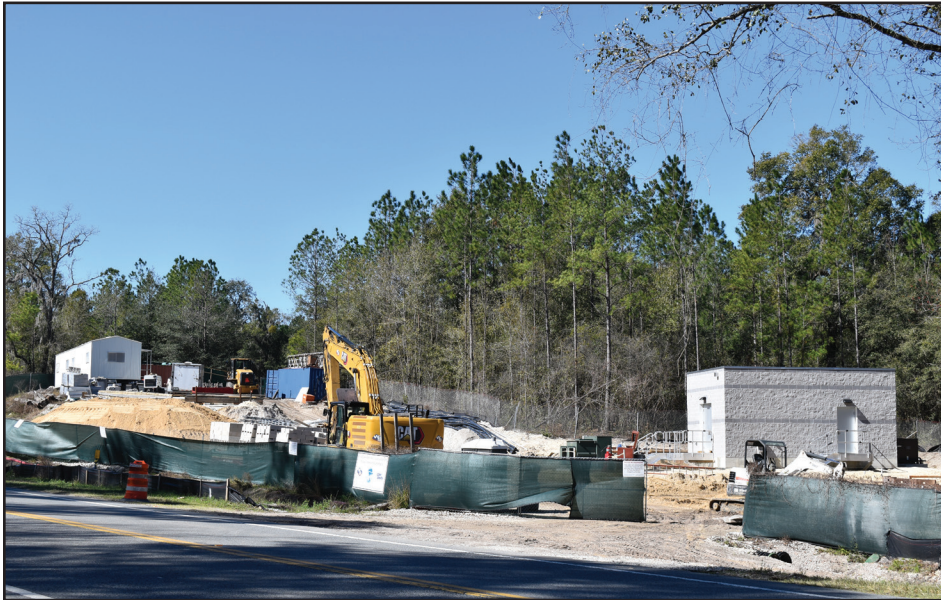
Work on the pump station for the Black Creek Restoration Project is moving along without any major setbacks. At the current pace, water should start flowing from the South Fork of the Black Creek into lakes Brooklyn and Geneva this time next year.
