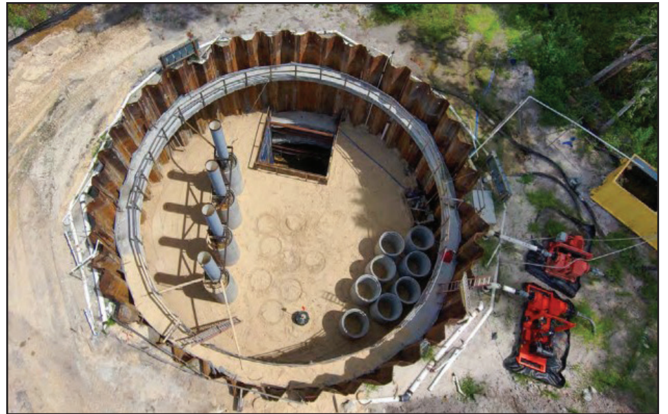
Crews have installed the underground pumps and a micro tunnel near the South Fork of Little Black Creek. The pumps have arrived at the warehouse and will be delivered to the site in the next three weeks.
