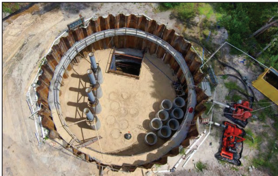
Crews have installed the underground pumps and a micro tunnel near the South Fork of Little Black Creek. The pumps have arrived at the warehouse and will be delivered to the site in the next three weeks.
