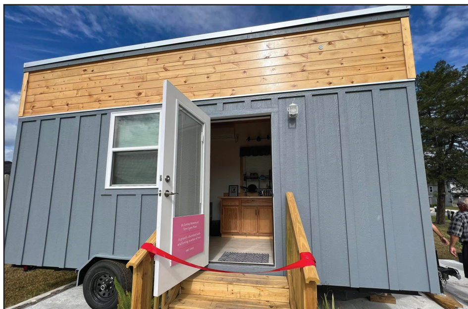
The first of eight tiny houses at Fort Barnabas needs plumbing and electrical work before the first homeless veterans can move in.
