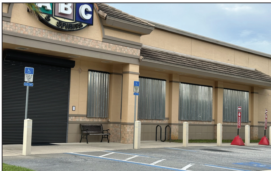
ABC Liquors on Fleming Island was one of 18 stops one company had to make on Monday to board up windows to reduce the threat of damage by flying debris.
