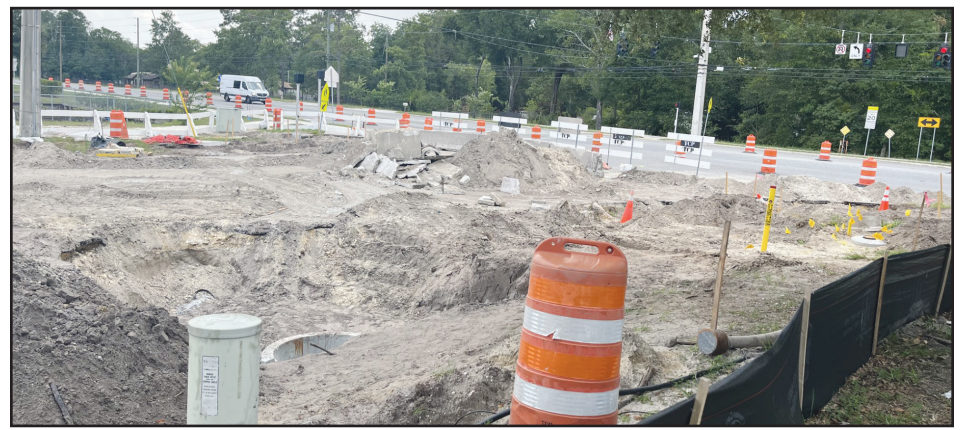
Construction at Henley and Sandridge roads will force many people in Lake Asbury to drive as many as 10 miles to buy groceries. Construction will last through the end of July.
