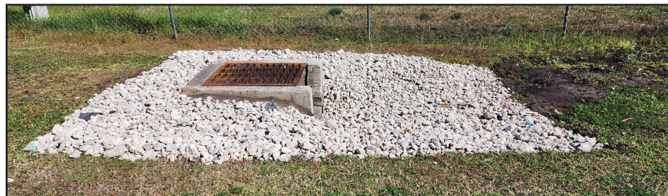
Drains have been cleared and rocks were installed to channel water from the parking lots.
