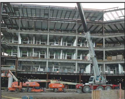
The final beam was put in place on Sept. 31, 2021. Fourteen months later, the hospital is ready to accept patients.
