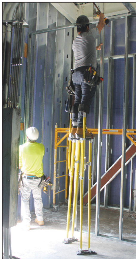
The first studs were installed on Sept. 2 as Grumpy's finally moves forward to re-opening on Nov. 21.
