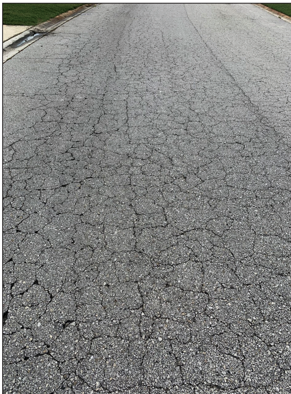
The county seeks to treat deteriorating pavement like this section of Harbor Island Drive.
