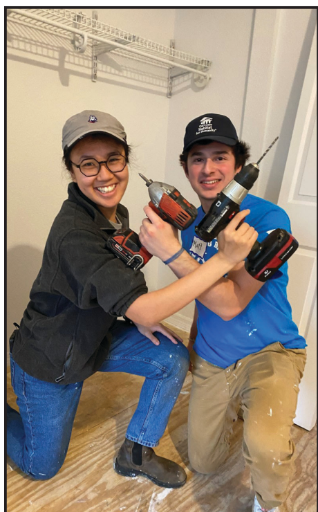
Two DeSales students found a way to have fun and move the new build a step closer to completion.
