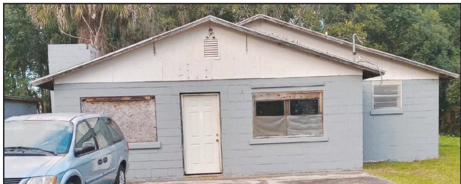
The current building at The Vineyard Transitional Center needs more than repairs. It needs to be knocked down and rebuilt, contractors said.
