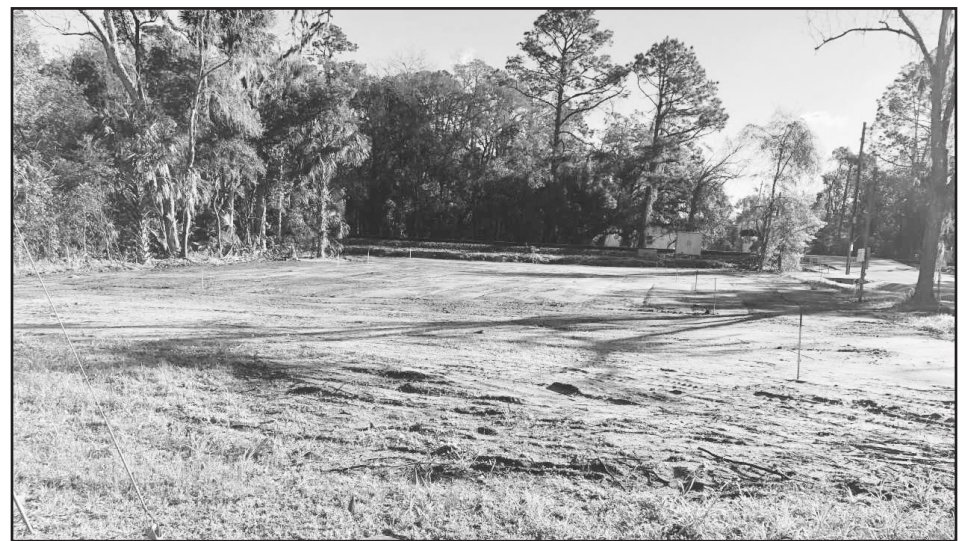
In a little more than a year, this empty lot was transformed into three homes in the Habitat Commons development.
