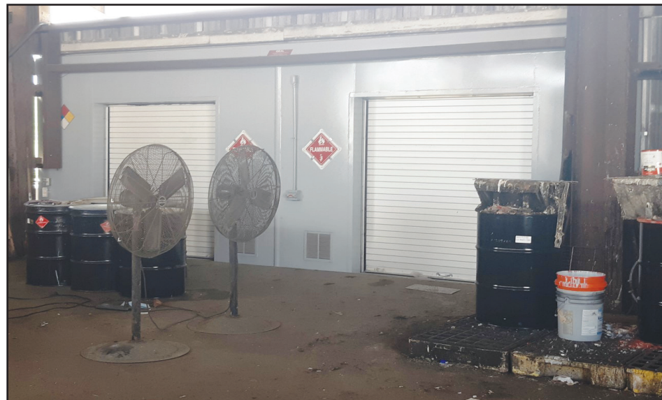
The three new hazardous waste buildings will help Clay County residents properly dispose of dangerous waste.
