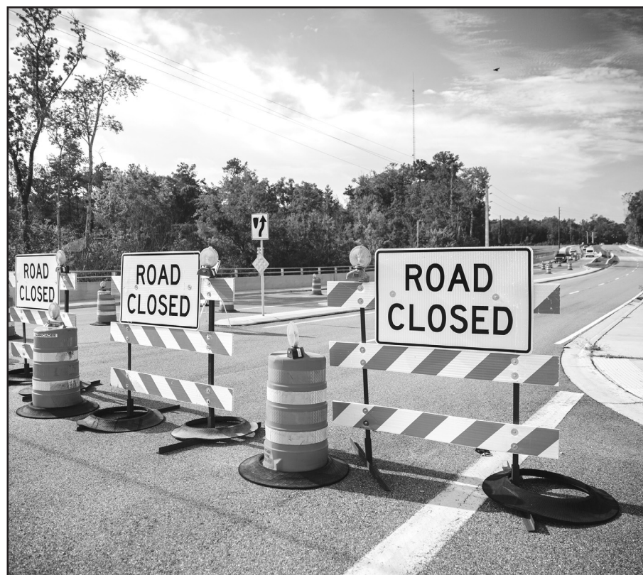
Signs and construction barrels block southbound lanes along Henley Road after county officials closed the lanes due to the road's lateral movement. The county is currently involved in talks with the engineer and contractor to figure out how to stabilize the roadway.
