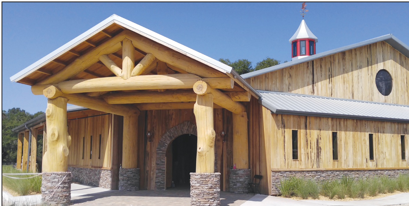
Tree trunks help form the entrance to Boondocks Grill and Bar in Lake Asbury, where construction is nearing completion.
